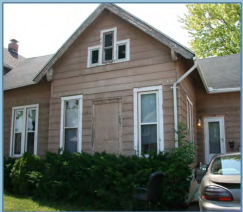
Long term Boarded-up front door
